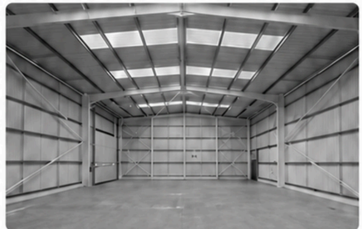
Pipe Bracing System
