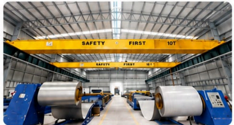
TOP RUNNING CRANE SYSTEM
